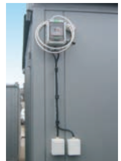
Detail of electroinstallation.
